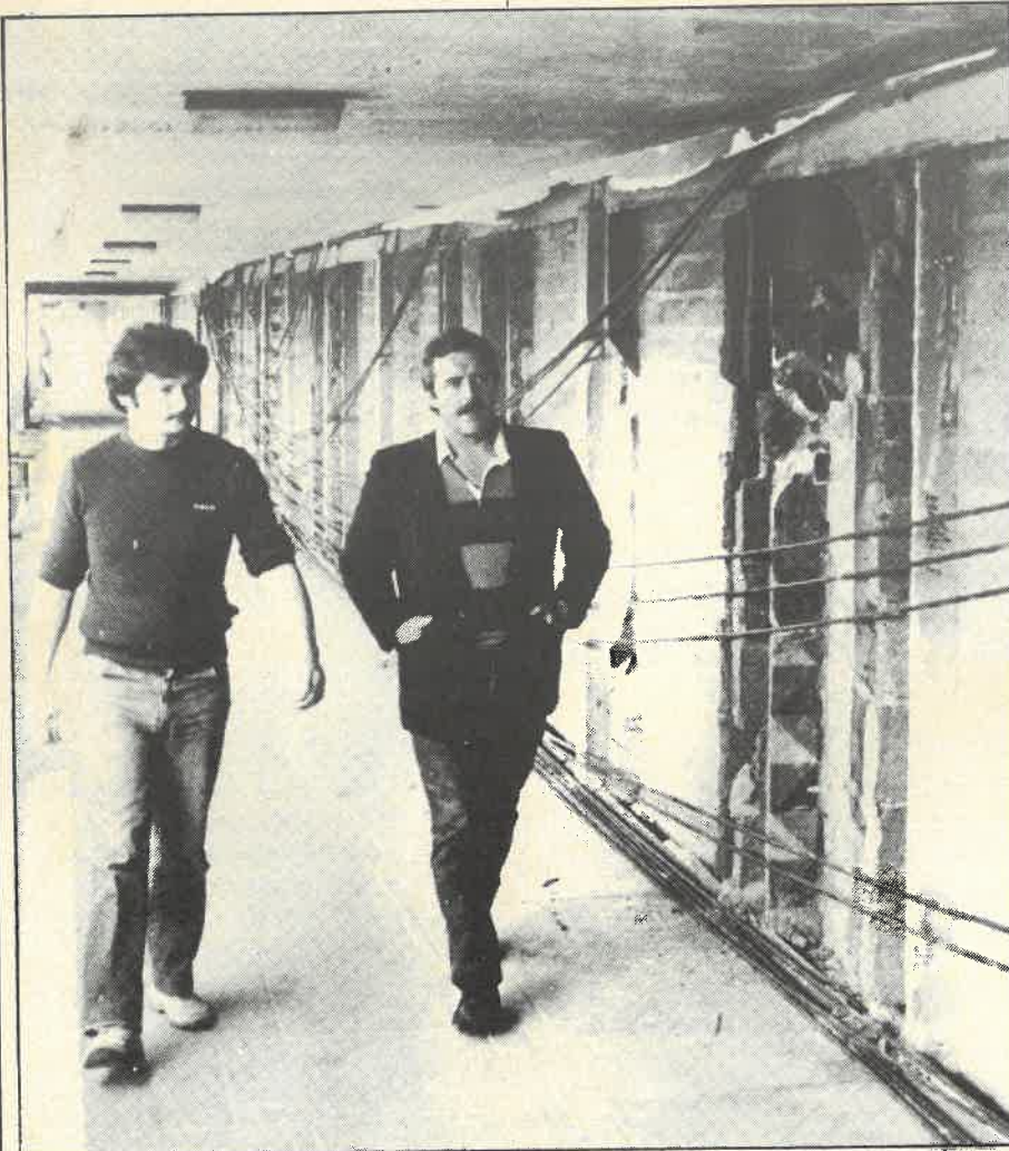
● Sinn Fein community workers inspect exposed live electricity cables along Divis' Whitehall Row — an obvious danger to local children
