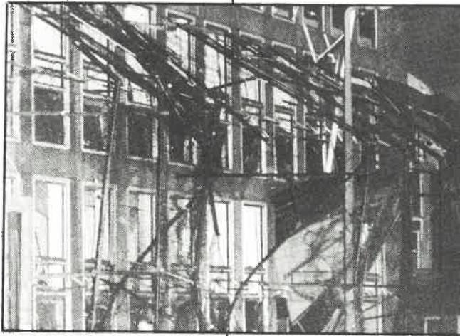
● Severe damage was caused to Belfast Law Courts in an IRA bomb on January 9th
